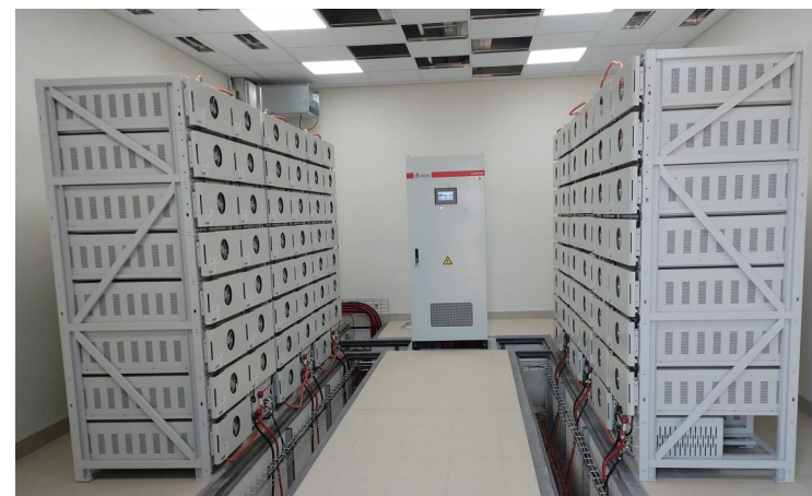
South Africa 1.2MWh
